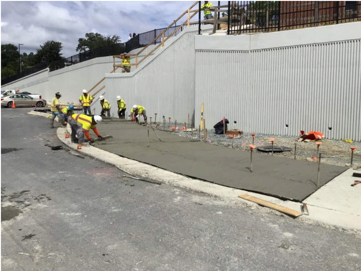
Restored sidewalk on the north side of Wayne Avenue and follow signage and crossing guards' directions. Image Source: PurplelineMD
